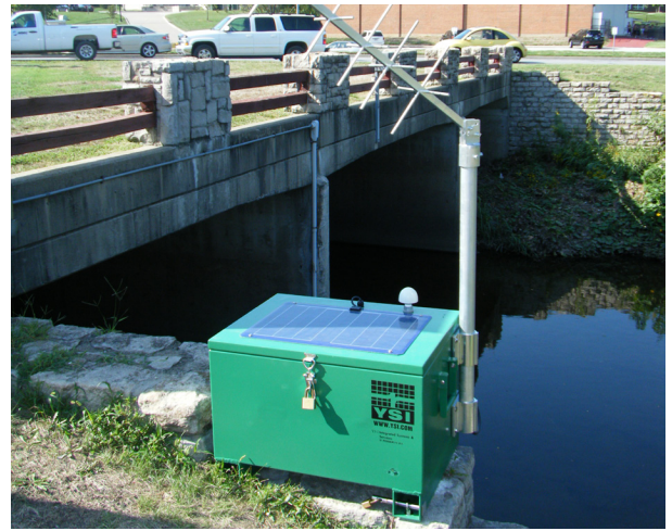
Portable water quality stormwater site in Kansas equipped with WaterLog GOES satellite data delivery, EXO water quality instrument and solar power.
