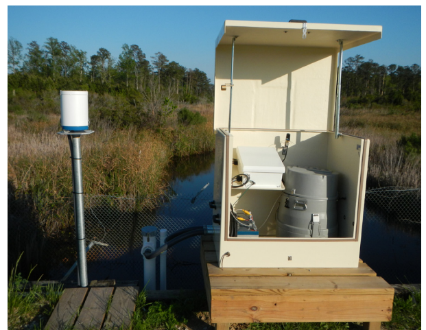
YSI Systems Stormwater monitoring enclosure with solar power, automated water sampler, cellular based real-time data/event notification, Waterlog rain gauge, EXO water quality instrument and a SonTek IQ flow sensor.
