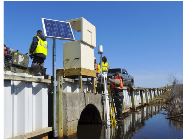
YSI's field services crew finalizing the installation of complete stormwater site in North Carolina.
