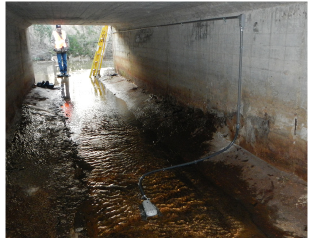
SonTek IQ acoustic Doppler profiler based open channel/non-full pipe flowmeter being installed in a typical stormwater culvert.
